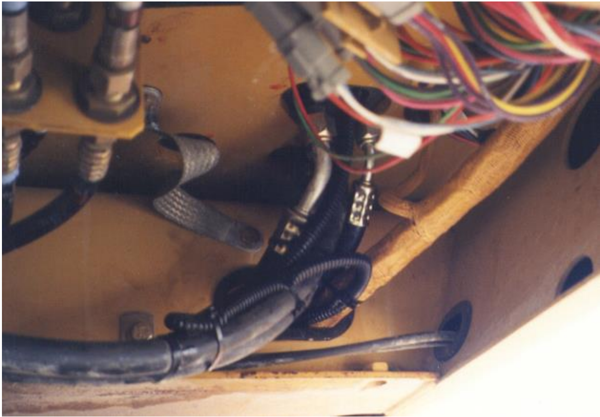
View showing underside of evaporator area with hose assemblies and drain tubes.
